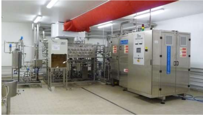
Figure 1. Tubular heat exchanger (left) and RF equipment (right)
